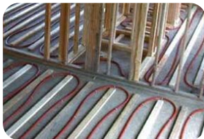
Radiant Floor Heating
